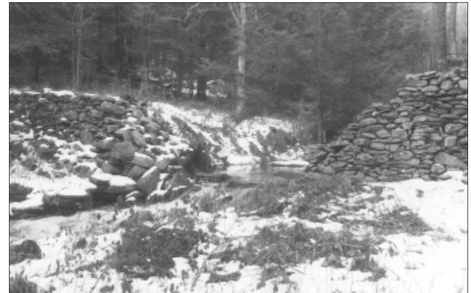
Breached Hutchinson's Hollow dam.
