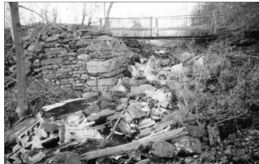
A portion of the breached Weed's Dam seen from the west side. The dam provided the volume necessary to operate the two waterwheels that powered two sets of blowing tubs for the blast into Weed's Furnace.
